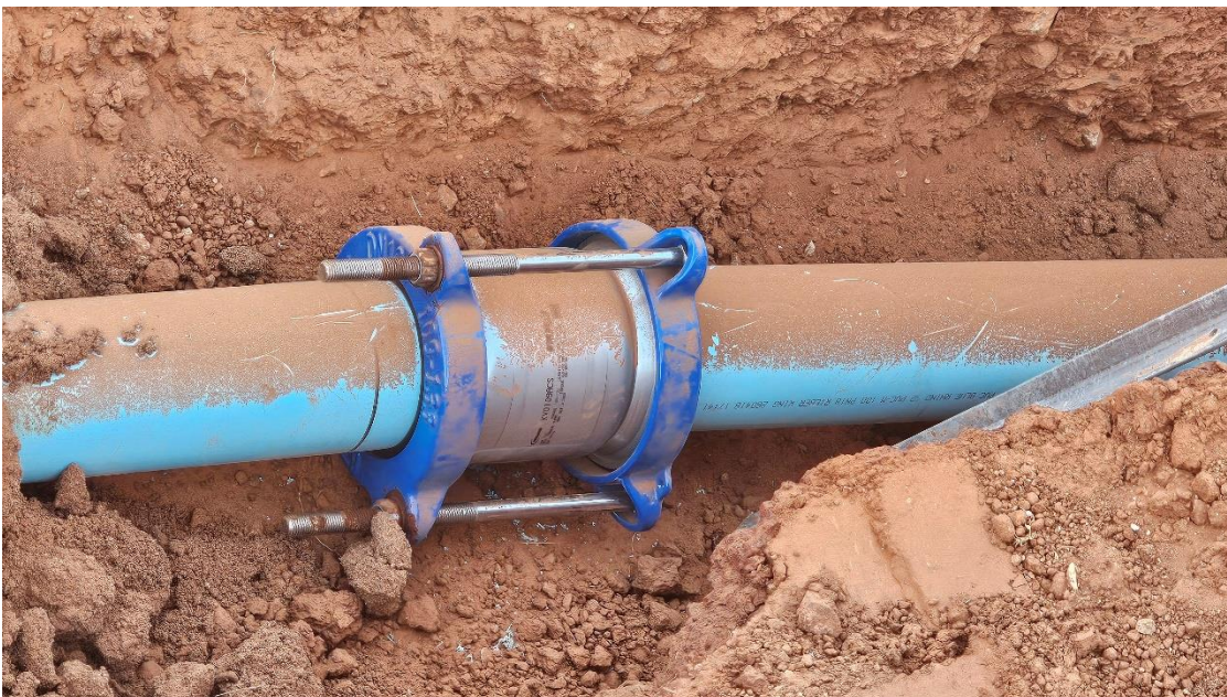
Sams St -Town water installation
